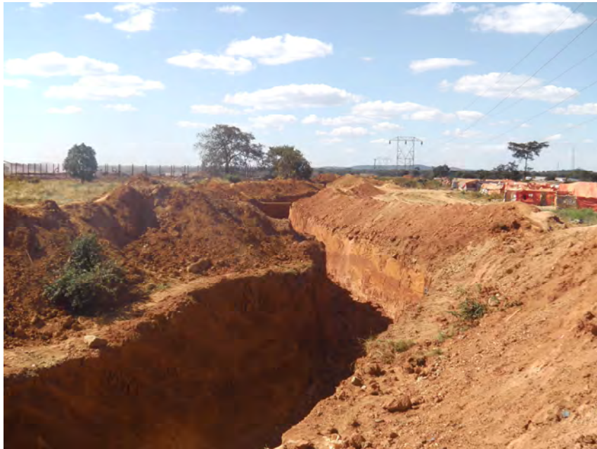
The trench in Luisha dug by Compagnie Minière de Luisha (COMILU), 20 April 2012 © Amnesty International
